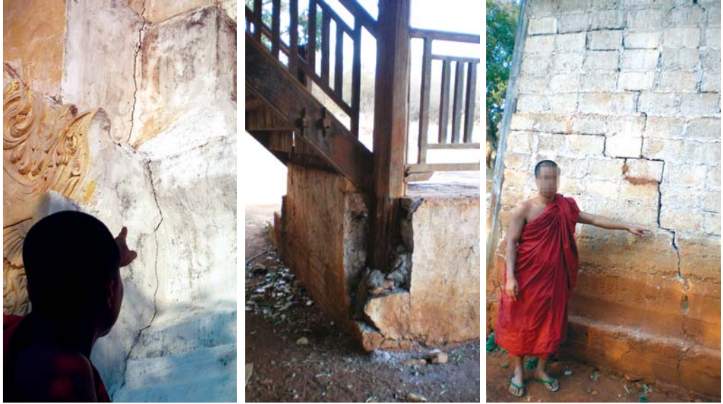
Local monks show temple walls cracked by explosions from mining for construction materials. Photos taken in March 2008
