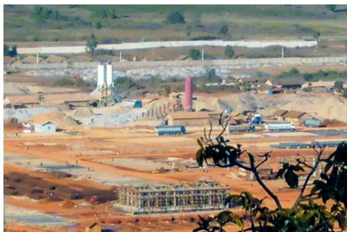
Construction inside the iron factory site. The wall around the site (in the background) has just begun to be built. Photo taken in December 2007
