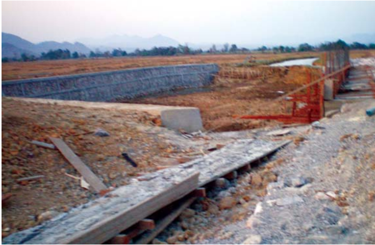
Construction of the factory pond blocked Thabet Stream and water has been diverted to the iron factory. Photo taken in March 2008
