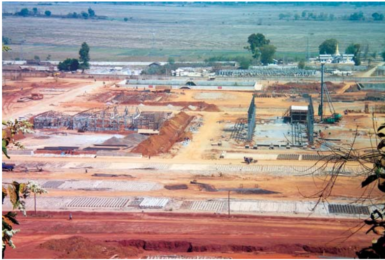
Looking east from the construction site of the iron factory. The pagoda in the upper right corner lies just outside the double wall around the factory. Photo taken in February 2009
