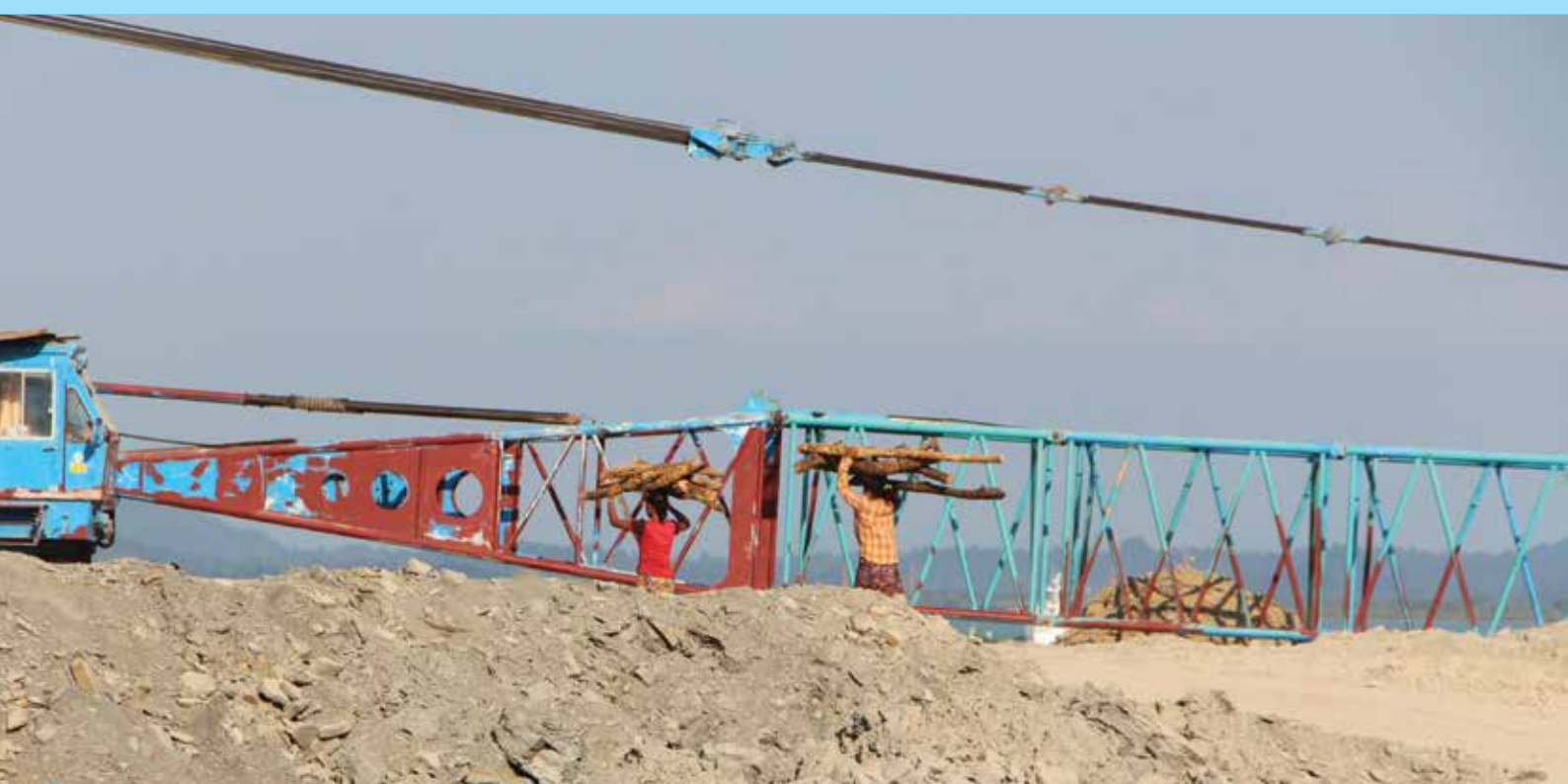
Below - Women carry firewood for cooking fuel at the deep sea port construction site, Maday Island.
